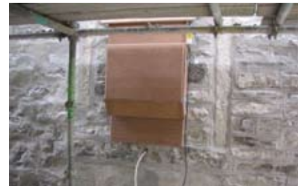
Newly wall-mounted box at a historic building refurbishment, Scotland
